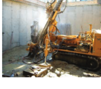
LEFT: The geology of the site made for a challenging geothermal installation.
