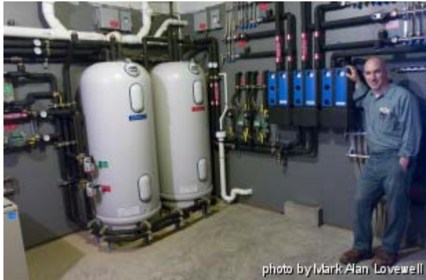
"This is where the love is," says Mr. Nelson of the heat pump.
