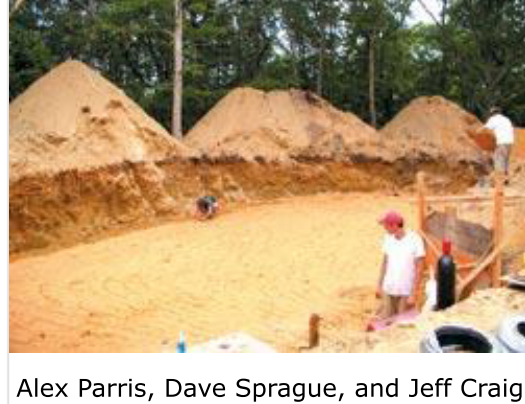
Alex Parris, Dave Sprague, and Jeff Craig Loops of copper tubing that will collect heat from the earth for a geothermal energy system stretch across a 2,500 square-ft. area where Alex Parris, left, Dave Sprague, and Jeff Craig put it all together. Photos by Janet Hefler
