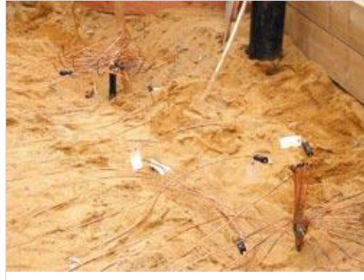
The intricate network of copper piping comes together in a manifold to carry solar-generated heat from the earth to the heat pump in the house. Photos by Janet Hefler
