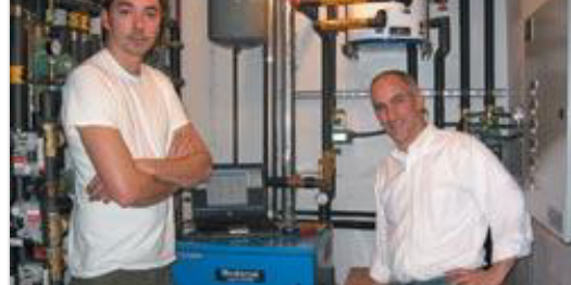
Dave Sprague and Brian Nelson Dave Sprague, left, and Brian Nelson tweak the settings for controlling the combination geothermal, solar, and conventional energy system in the home of Sarah and Bruce Nevin in Edgartown. Photos by Janet Hefler
